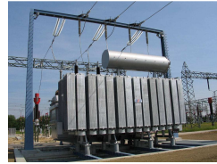
A: Lambach 200/200/30 MVA, 220/120/10 kV phase-shifting transformer
