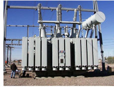
USA: Thunderstone 280 MVA, 230/70,8 kV Autotransformer
