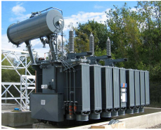
UK: Kettering 90 MVA, 132/33 kV Gridtransformer
