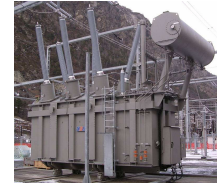
CH: KMW Stalden 125 MVA, 220/130 kV Autotransformer
